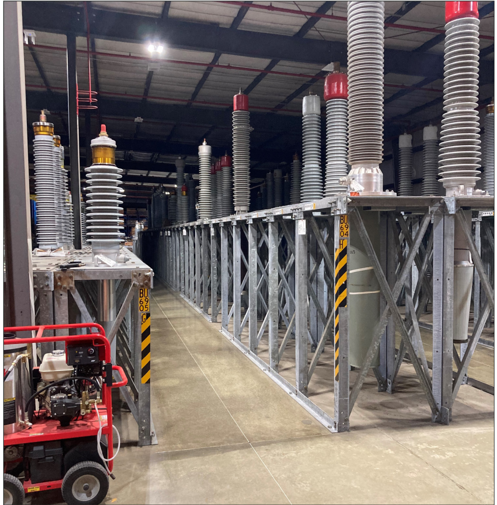
Figure 4: Spare Transformer Bushings Stored at a Utility Facility
