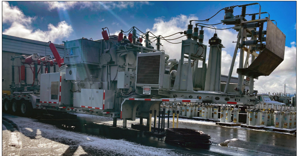
Figure 3. Example of a Mobile Substation
